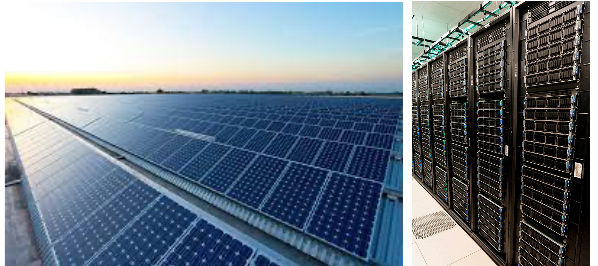
On-site computing facilities powered by solar plants
