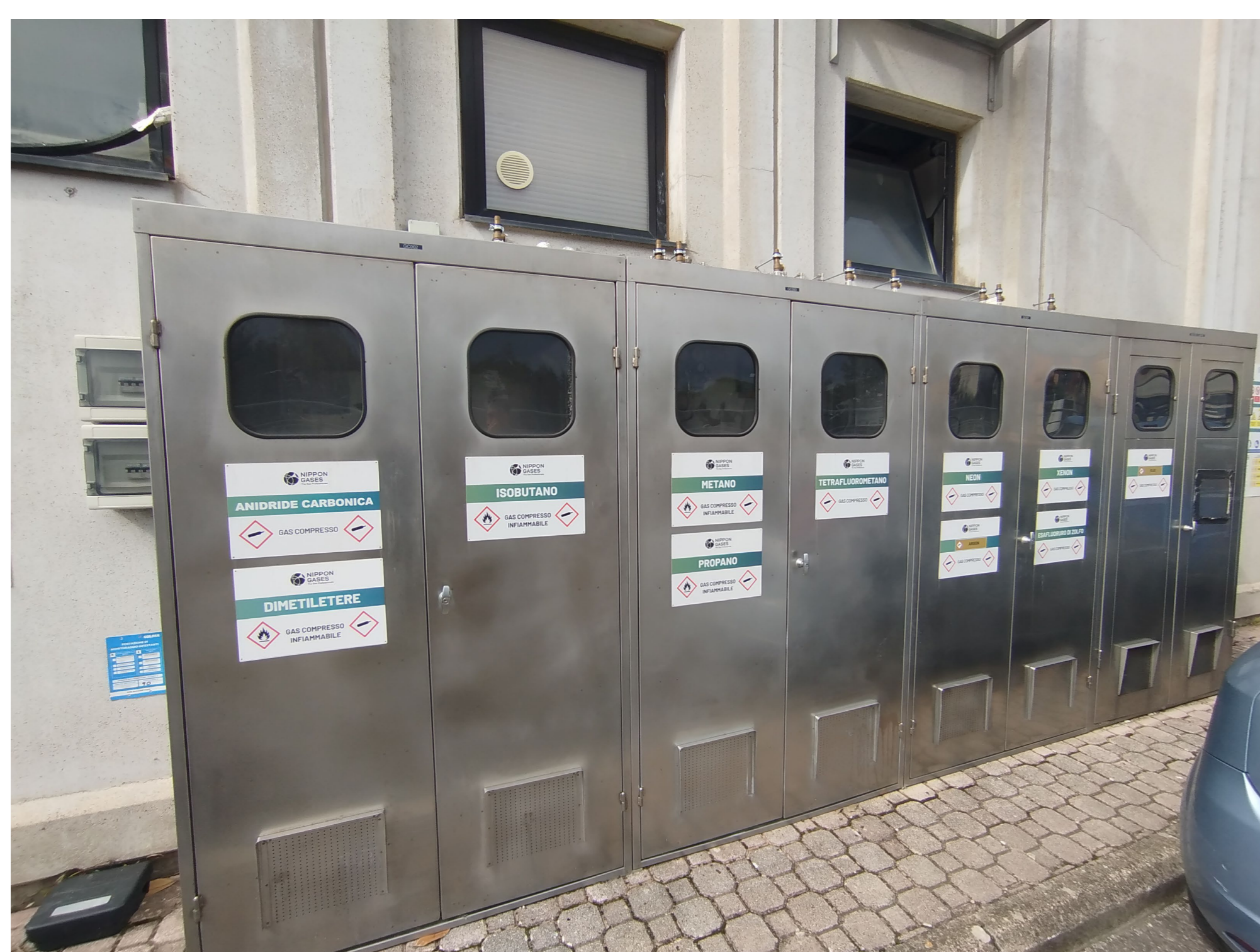
Fig. 3. The four gas cabinet hosting the 12 bottle of different gas to prepare the detector filling.
