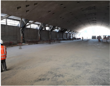
Each of the 6 “botti” (barrels) is ~5000m 2 of usable IT space
