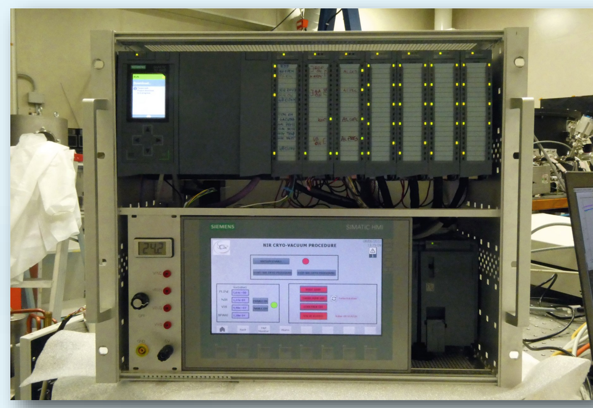
PLC Subrack (front view)
